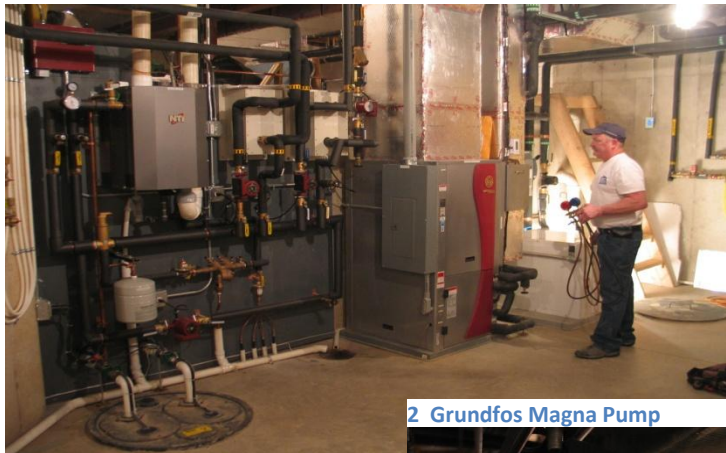
1 Main mechanical room
