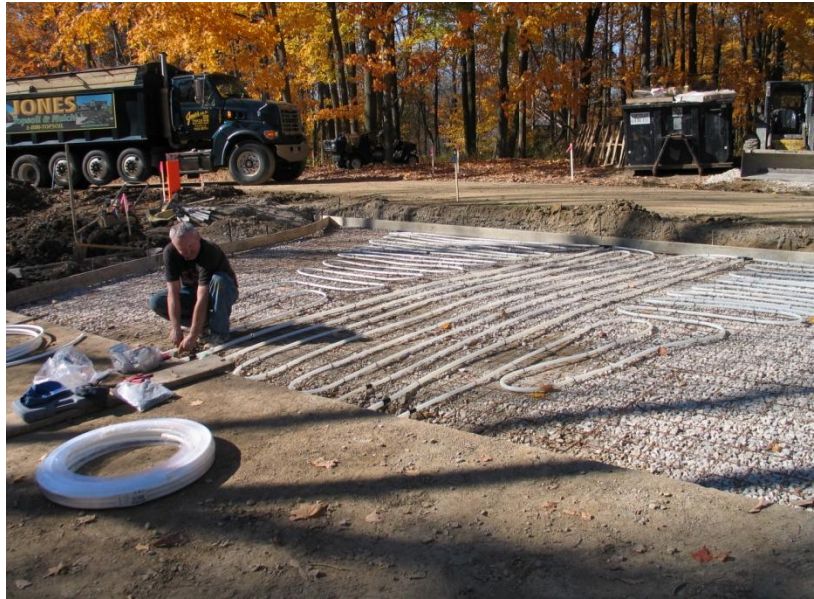
4 Driveway Snow Melt Piping
